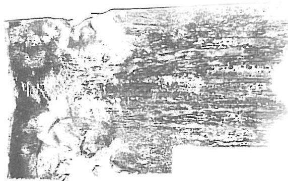
FIG. 1. As received failed section of chlorinator line showing extensive pitting, channels and perforation.
